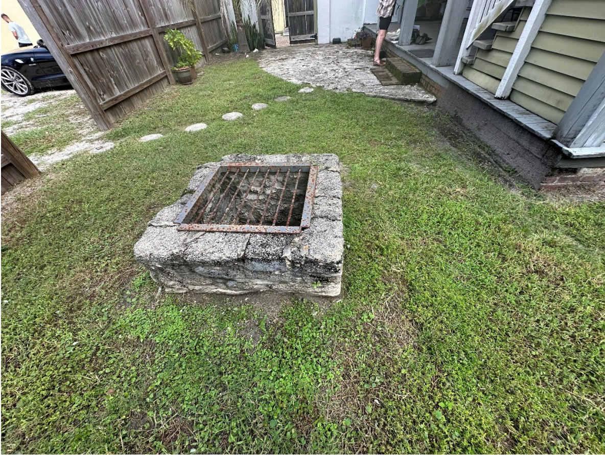
Figure 7. Yard view of the Watson House facing east. Note the masonry well, the concrete stepping stones, and the concrete pad in front of the porch.
