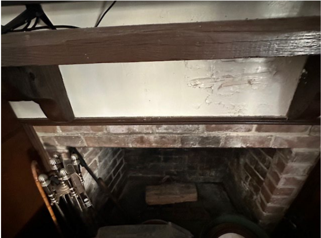
Figure 7. View of the fireplace in the second floor Living Room. Note the peeling paint below the mantel.
