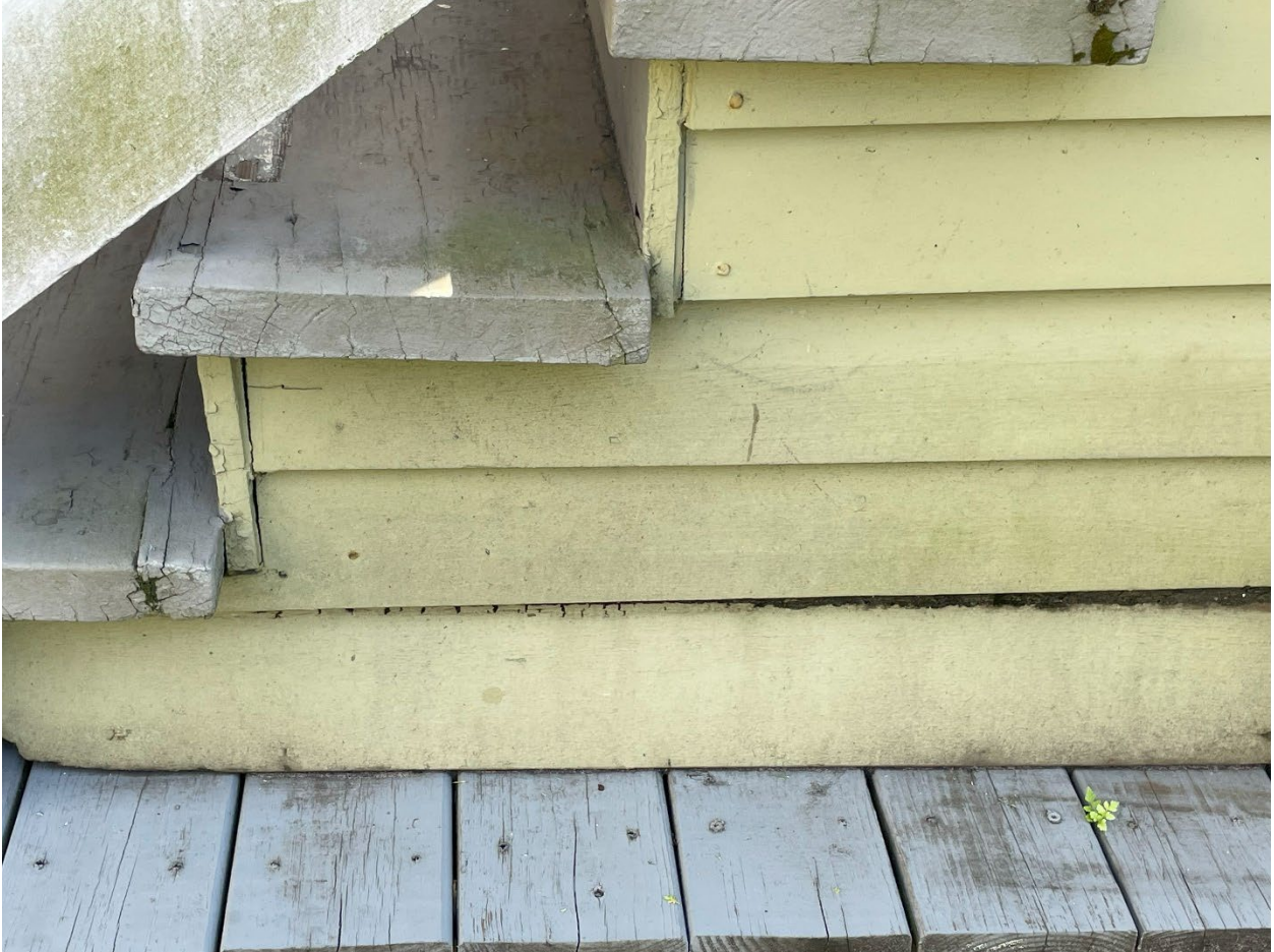
Figure 4. Low view of the exterior stairway on the porch of the Watson House. Note the condition of the steps, the siding, and the visible part of the railing.
