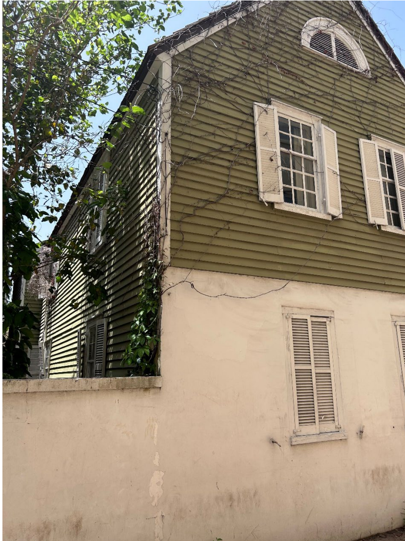
Figure 5. View of the east façade of the Watson House. Note the vines that begin in the southeast corner and run up the building to the exterior of the east side.
