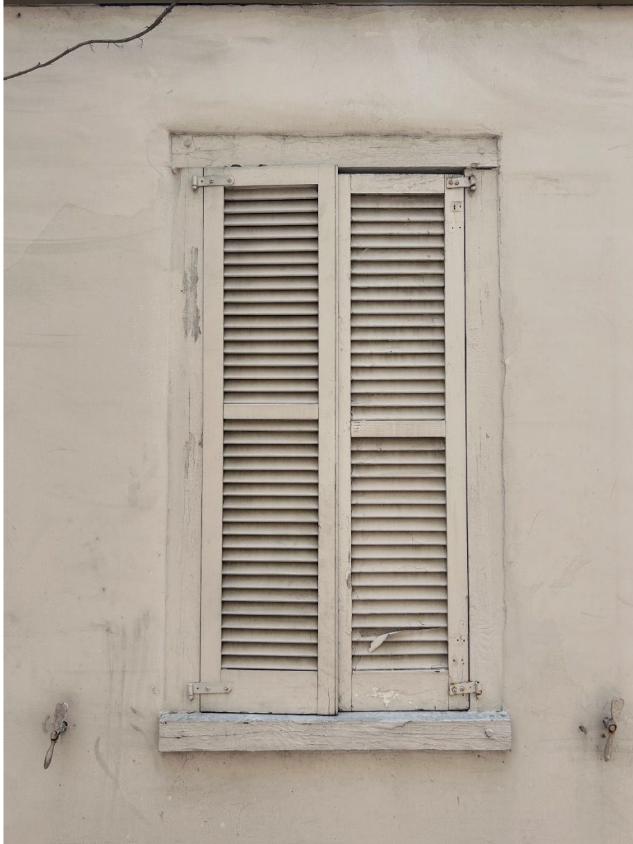
Figure 11. View of a first floor window on the east façade of the Watson House.
