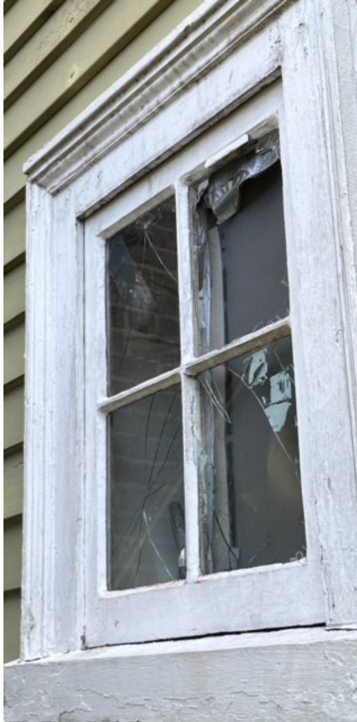
Figure 9. View of the broken window on the first floor ell of the Watson House.
