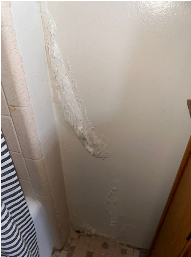
Figure 6. View of a blister in the wall of the second floor Bathroom. Note the proximity to the shower.
