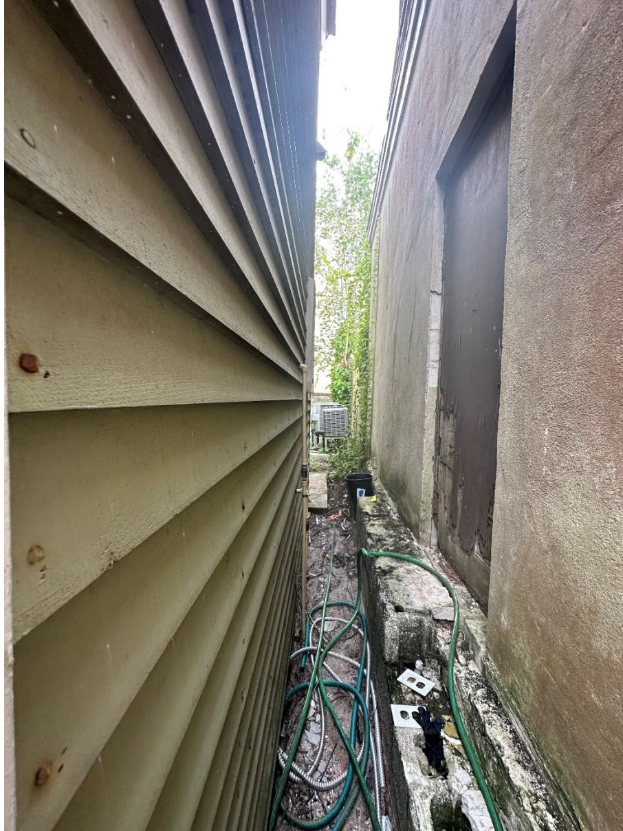
Figure 5. View of the south boundary of the Watson House property. Note the neighboring building to the right.
