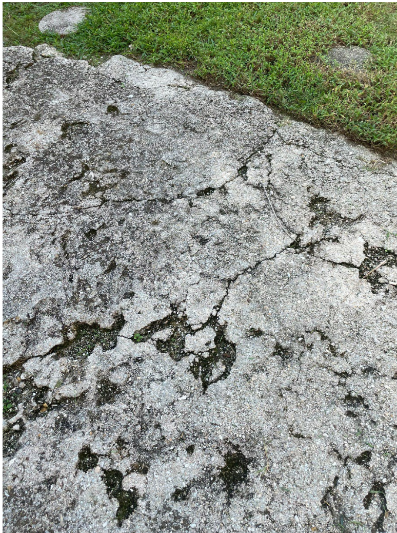
Figure 1. View of the concrete pad that leads to the porch of the Watson House.
