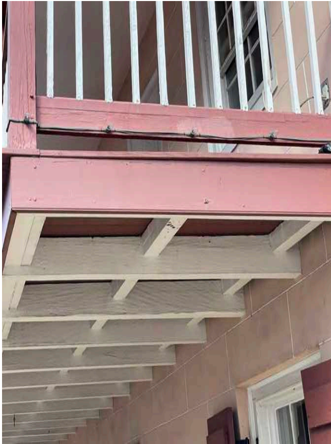
D: West Wing, Balcony, looking NE and up
